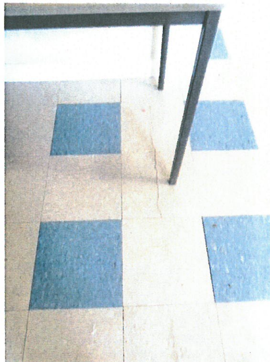
Photograph 6 – Cracking to floor tiles
