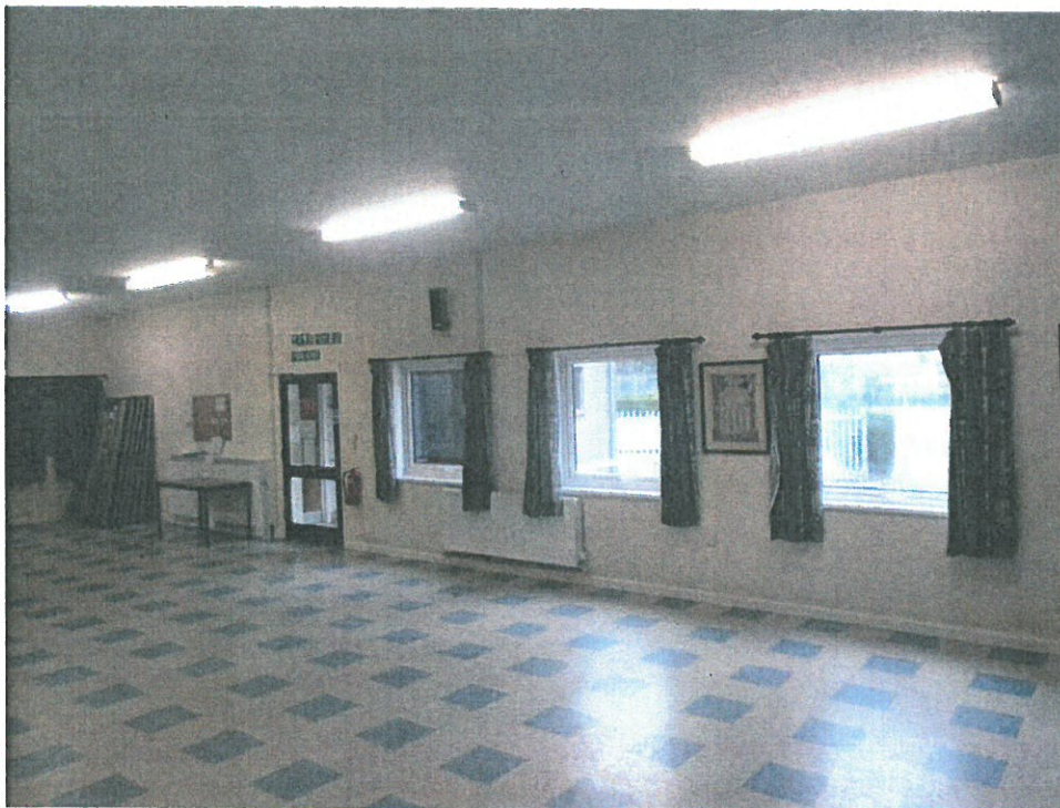
Photograph 14 – Long wall with large openings and likely insufficient butressing
