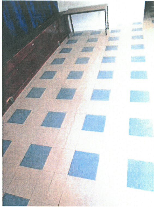
Photograph 5 – Cracking to floor
