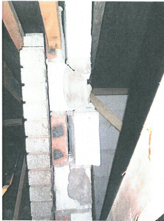
Photograph 13 – Loose block in attic
