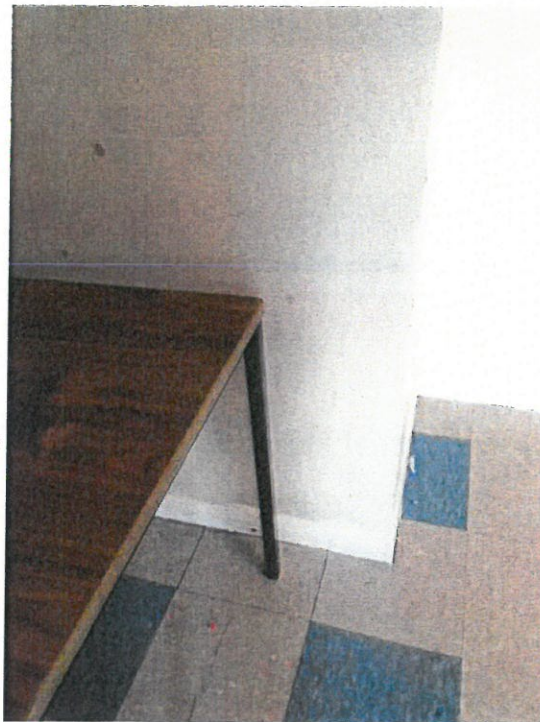
Photograph 4 – Cracking to internal wall
